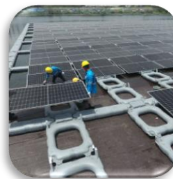
Floating Solar Power Plant
