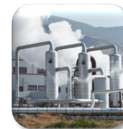
Geothermal Power Plant
